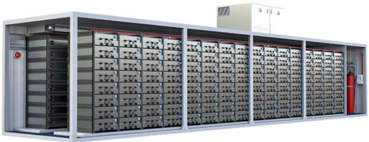
Figure 1: Li-ion battery energy storage system with integrated fire protection system
